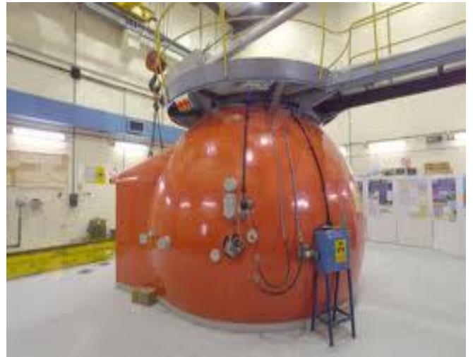
Fig. 1 - TAPIRO reactor room.
