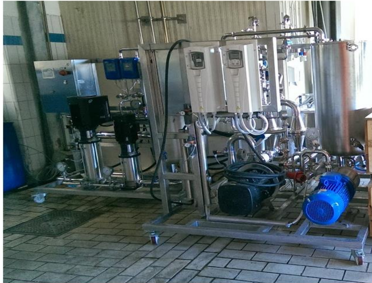
ENEA plants at milk production plant in Apulia: PON project Be & SAVE, 2015
