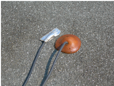
Fig 1. T1 and T2 probes on the roof
